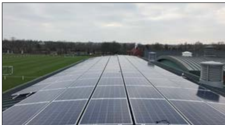
Solar panels on roofs of Dulwich College
